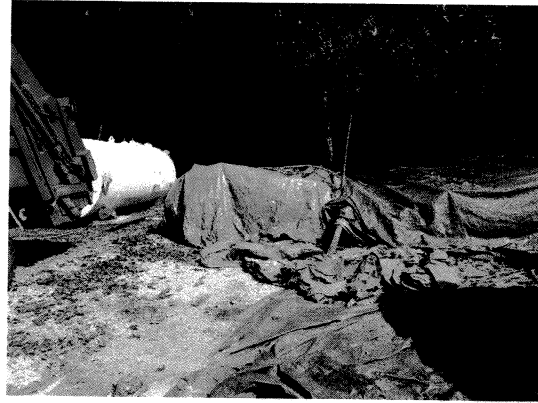
Water Pipes and Filter Tank
